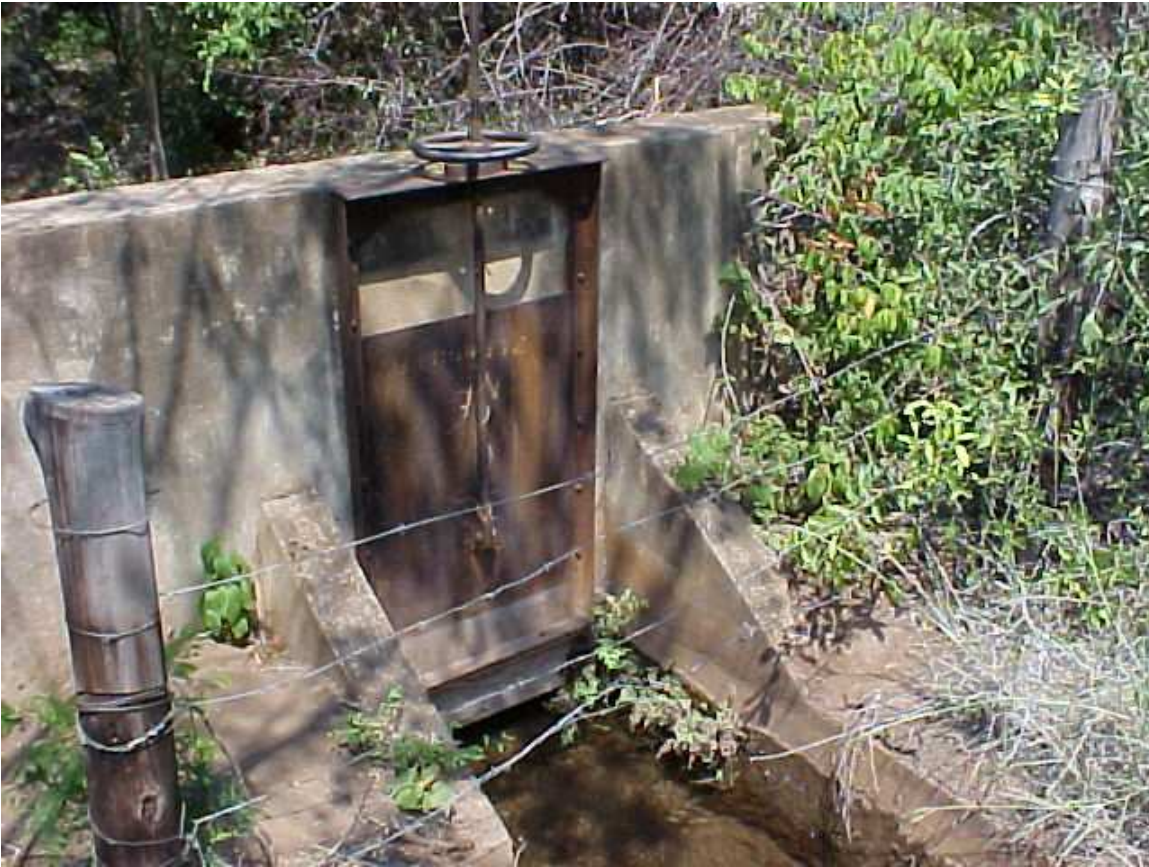
Figure 7 – Example of an adjustable gate which is able to regulate the water flowing into the principle canal. The gate and all its components should ideally be galvanised.
