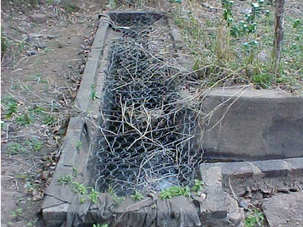
Figure 14 – Intake to 100m buried pipe. The canal may be seen to be coming in from the right.
