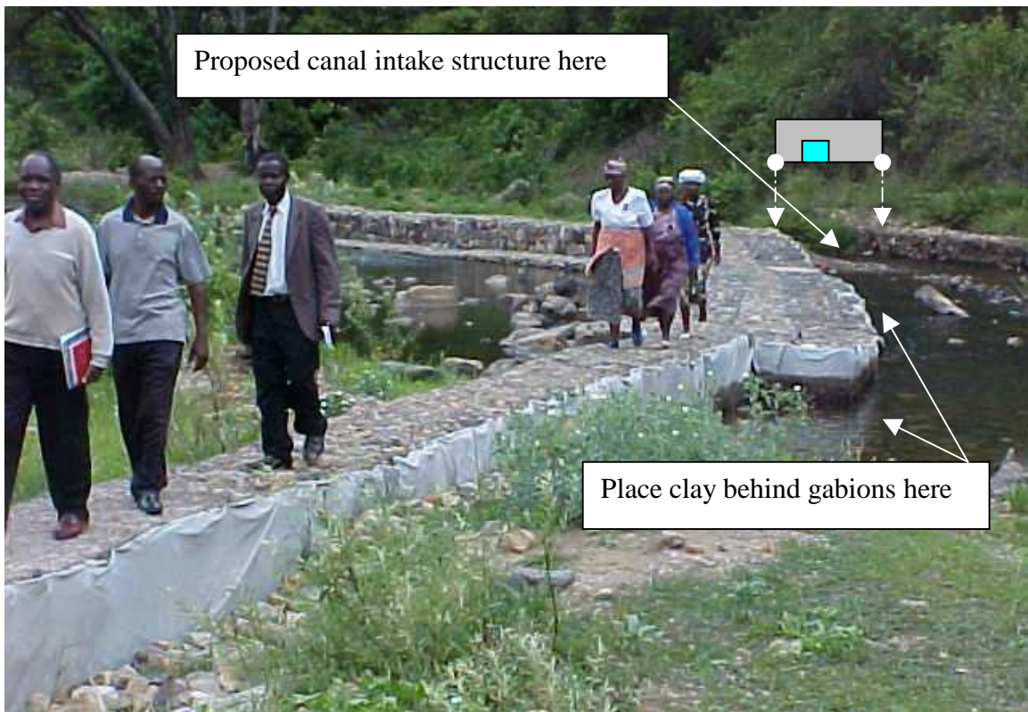
Figure 3 – A view of the gabion structure built by the community in July 2003 with material supplied by the Lebowakgoma offices of the Department of Agriculture. Some of the community leaders are in picture. The geofabric may be seen on the upstream side of the weir, and decomposition from UV attack will accelerated after 2 yrs.
