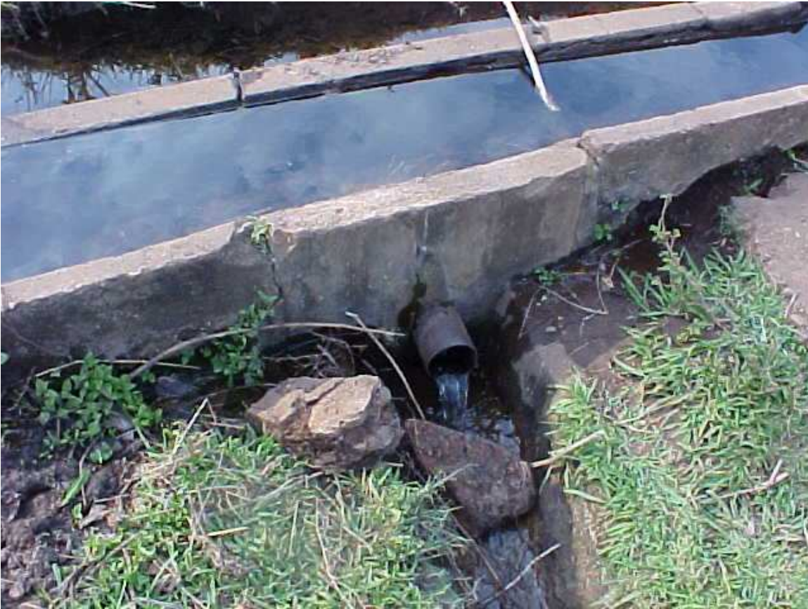
Figure 15 – View of gate 1. Water flows from the primary canal (background) into the secondary canal by means of an 80 mm galv pipes. (In this picture the flow is slow as the pipe has been blocked with a plastic bag and rock on the other side – see figure 9).
