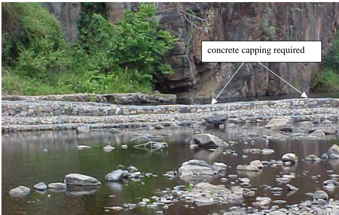
Figure 4 – the top of the weir is not horizontal – with undulations of approximately 200mm, which may be corrected by applying a concrete topping
