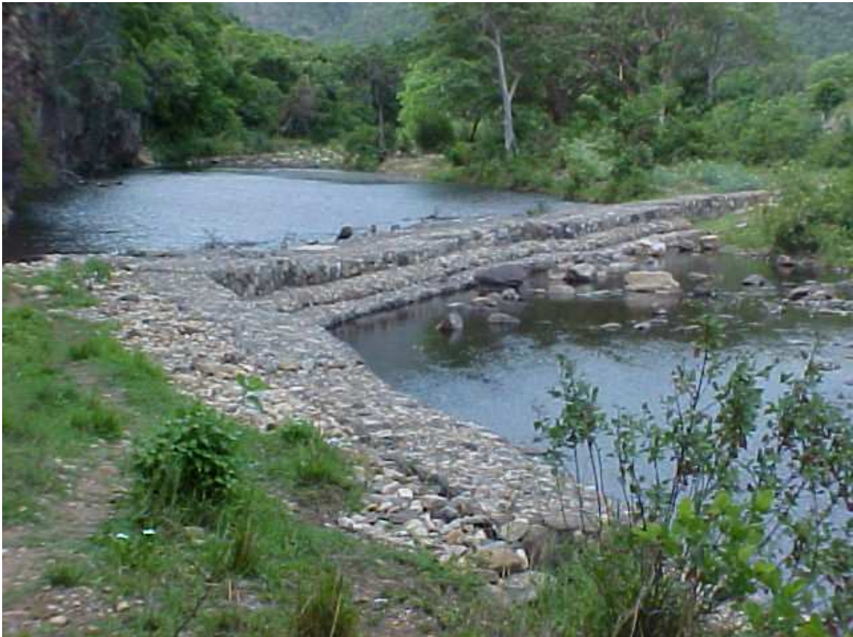
Figure 1 - Gabion Weir as seen from the west bank - built by community and LDA
