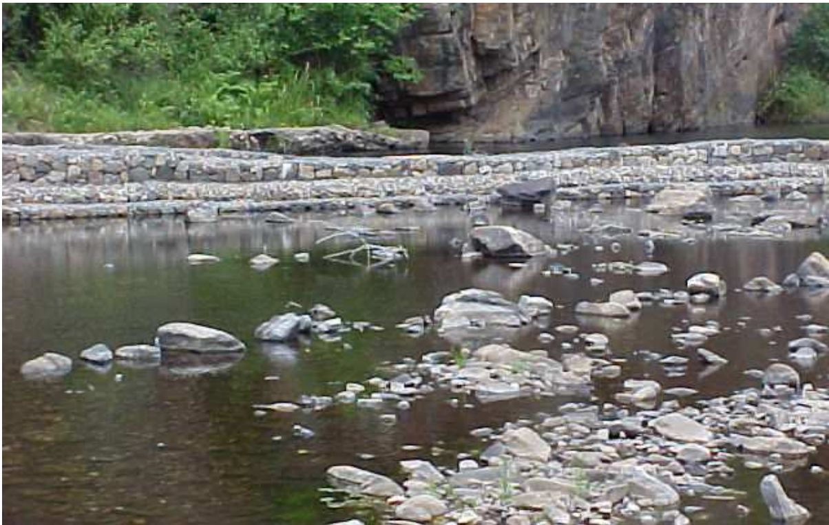
Figure 3 - Upstream view of gabion weir – the water in the river passes directly through the gabions, and virtually no water goes into the canal.
