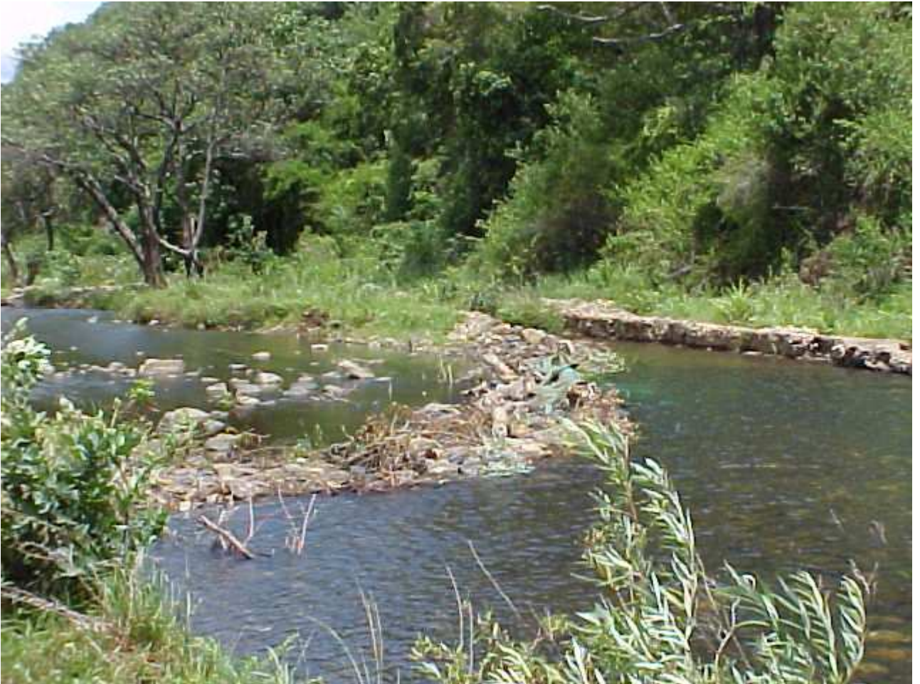
Figure 2 – The flood damage to the diversion weir is evident. Water currently percolates freely through crude rock/soil makeshift structure. The upstream level should be approximately 400mm higher than at present in order to divert enough water into the canal. The mouth of the canal is out of view, but is to the top centre of the picture.
