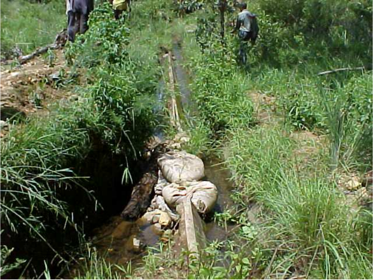
Figure 4 - The upstream level is too low to make the water flow in the canal. Notice how the supporting material has been eroded because there is no barrier wall at the start of the canal.
