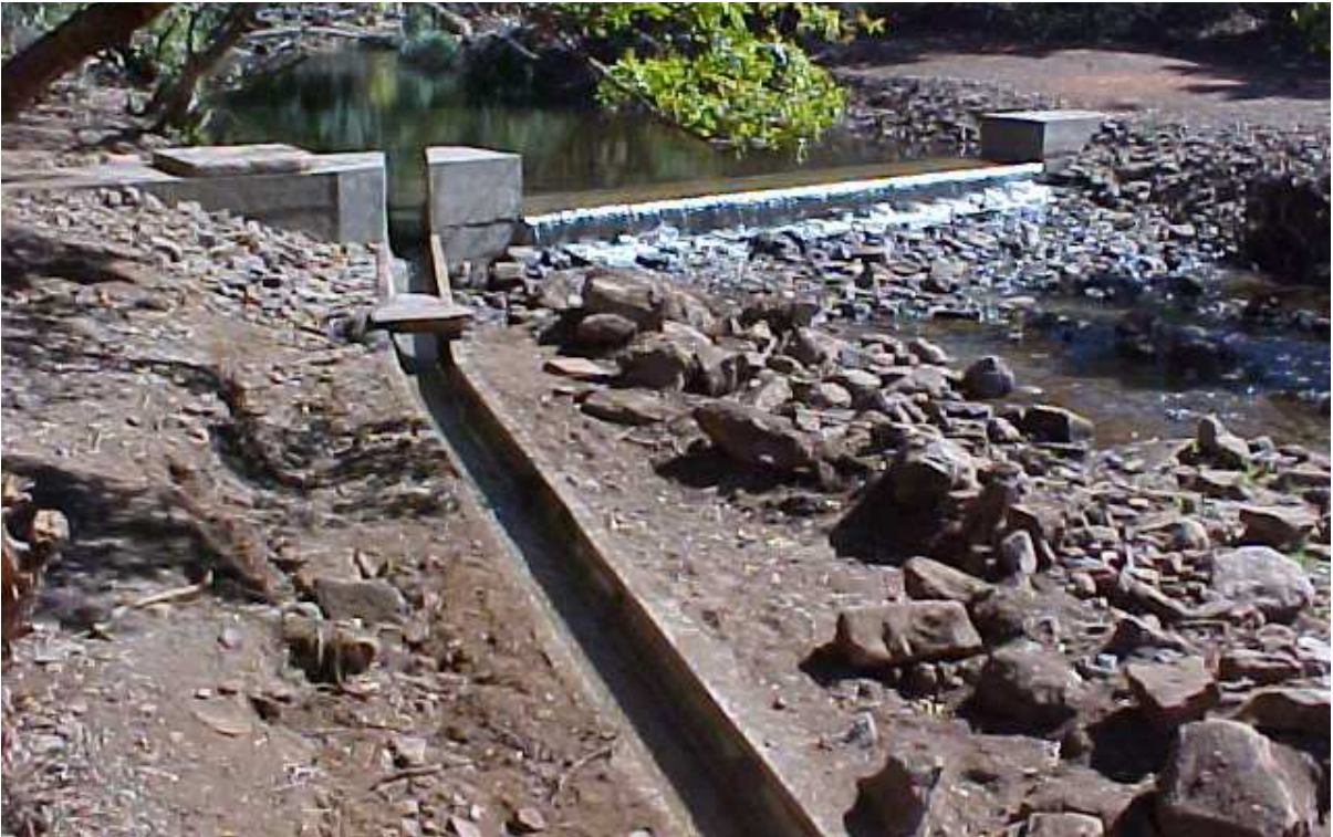
Figure 6 – The diversion weir and sluice gate off-take at the start of the 7km canal at GaMathabatha (about 40km from Fertillis). The weir and this section of the canal were built by DFA in July 2003 and are additions to an existing 7km canal.
