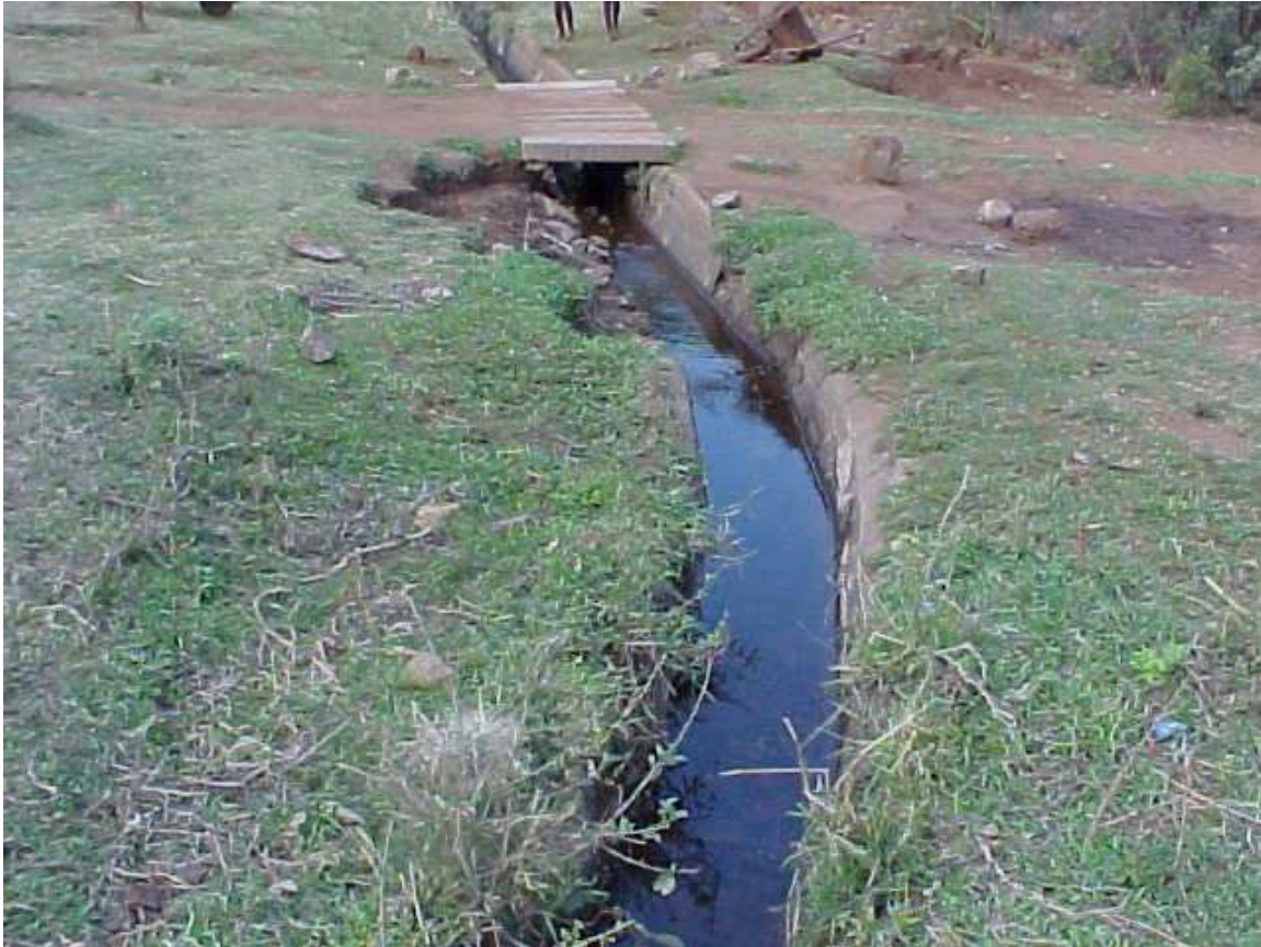
Figure 12 –A broken left shoulder, just before the bridge, necessitates a ‘major repair’
