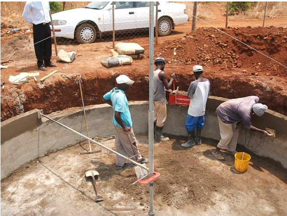
Figure 6 – A ‘Finnbuilder’ traveling mould in operation. Notice the pole/arm nearby which is used to keep the Finnbuilder in the correct ‘orbit’. Notice too the floating process underway which does away with the need for subsequent plastering operation.
