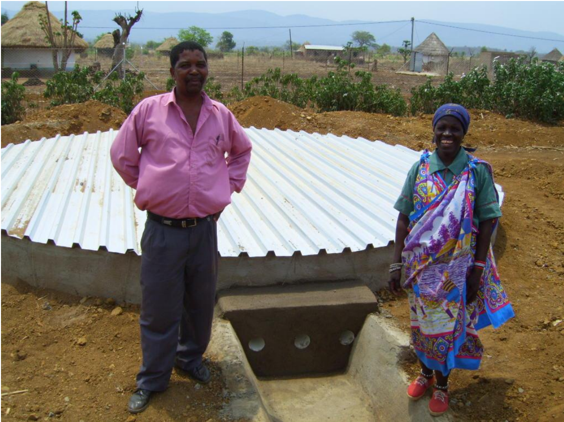
Figure 5 – A completed Standard dam – on the day of handover to house owner Muthavhini
