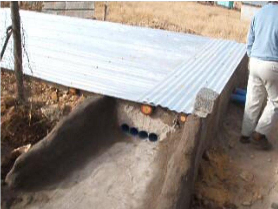
Figure 15 - Inlet structure for the box chamber
