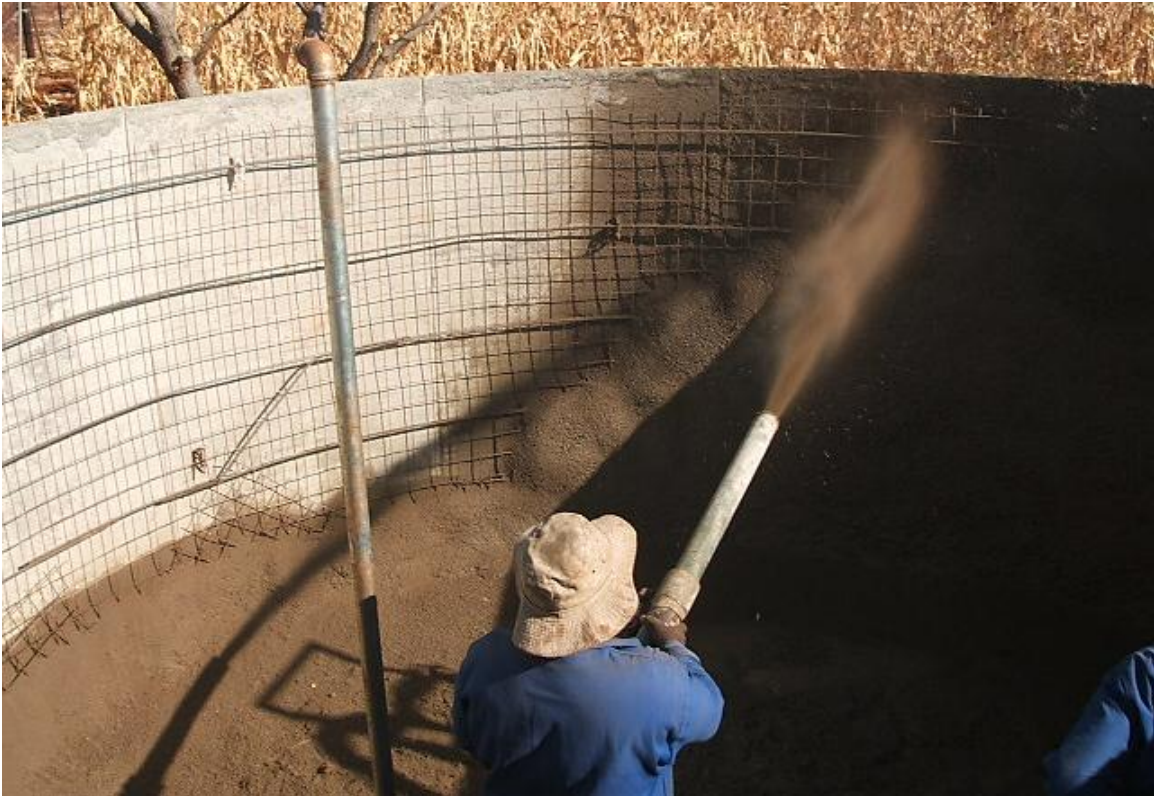
Figure 7 – Shotcrete being applied to the shell of a gunite dam. Note the Y10 hoop steel, held in position by the ref 100 structural mesh.
