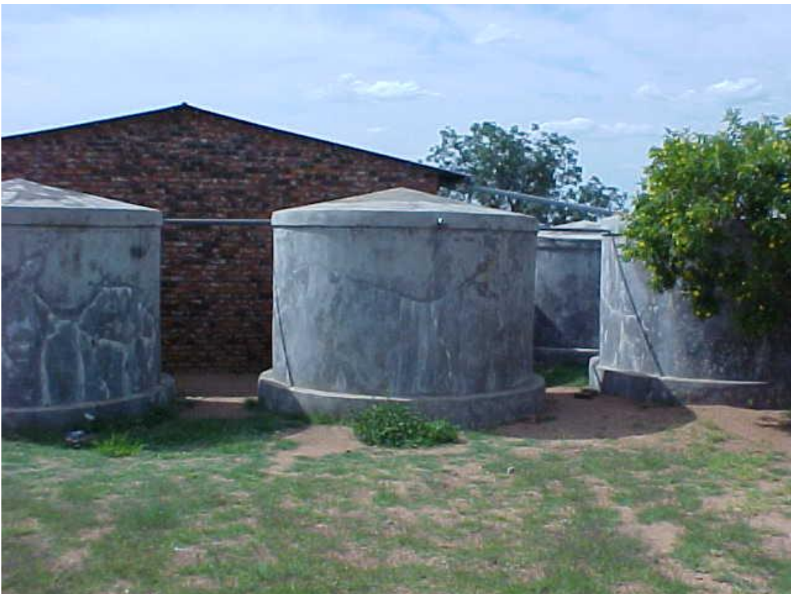
Figure 8 – Example of above ground ferro-cement tanks – the tanks are less than 3m diameter.
