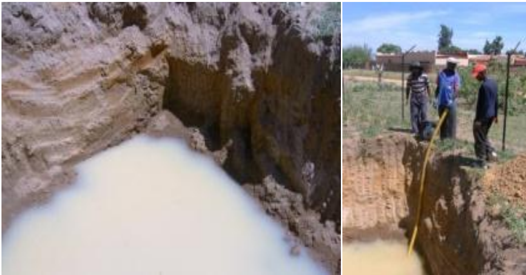
Figure 1 – A view of the inundated excavation
