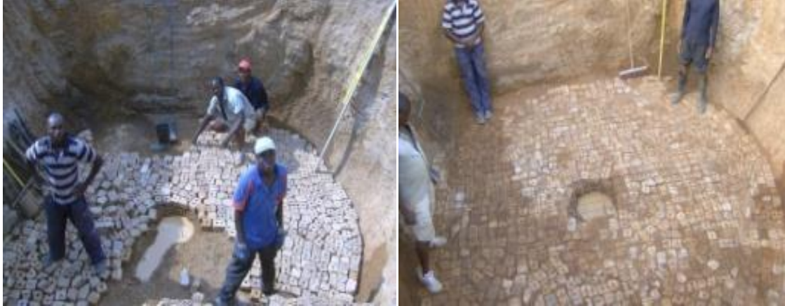
Figure 2 – Drainage layer consisting of broken bricks, with spaces filled in with sand/gravel.
