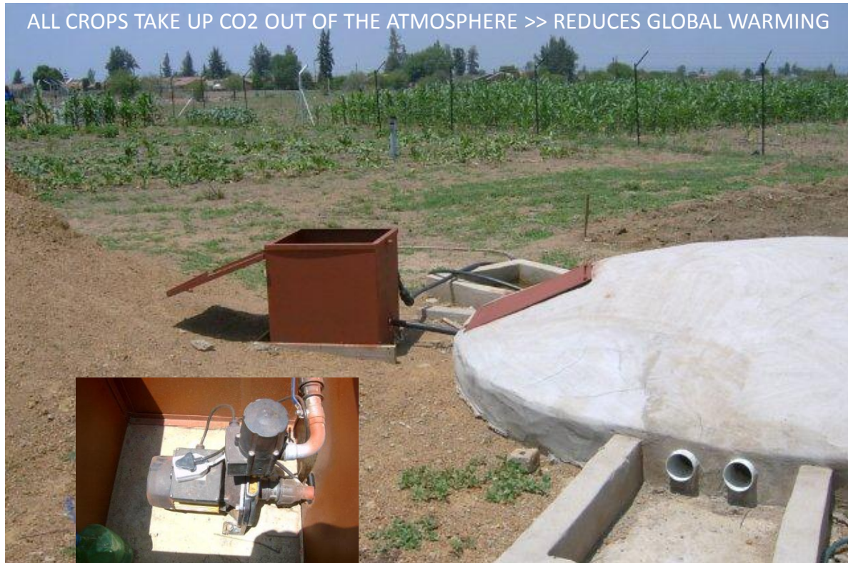
Figure 14 – The completed ferrocement RWH cistern showing the irrigated crops in the background.
