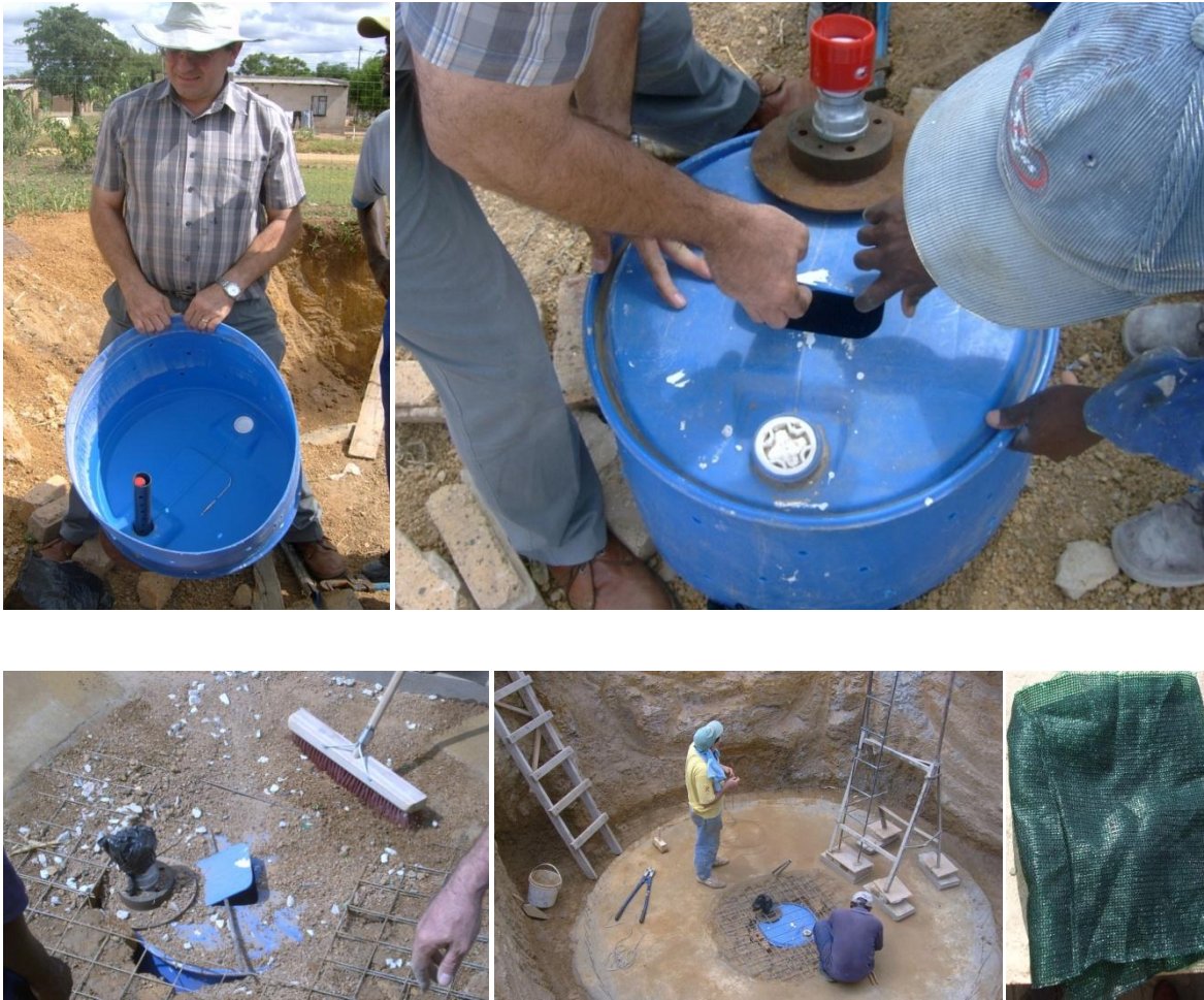
Figure 4 – Clockwise: (a) a plastic drum cut in half, with the filter/suction pipes protruding through; (b) a hole is cut into the lid of the drum to allow grit to be poured inside; (c) gravel is swept into the cavity, and around the drum; (d) the opening in the reinforcing is repaired; (e) the NRV is covered with filter fabric.
