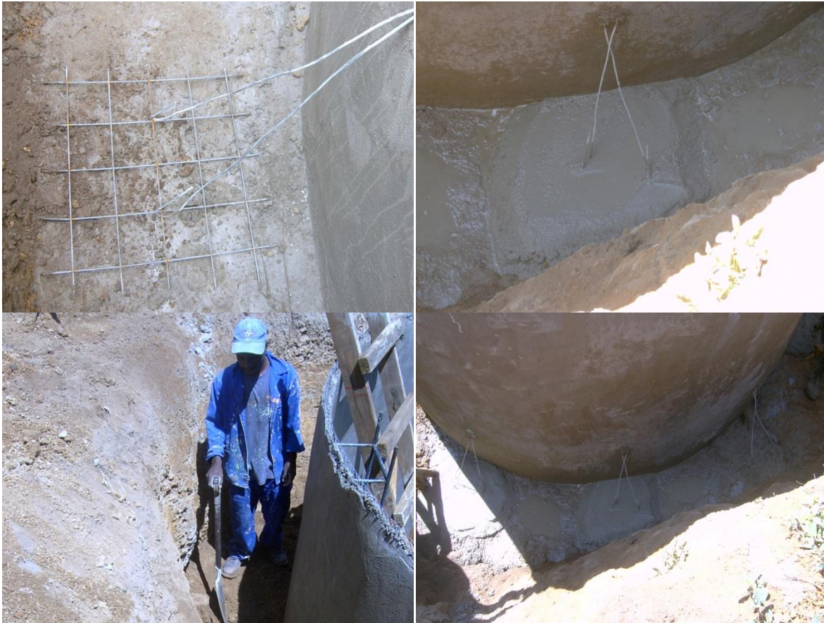
Figure 12 - Reinforced concrete anchor pads are constructed around the circumference of the cistern and are anchored to the walls. Once the backfill has been placed and compacted, the tanks is effectively restrained from floating out the ground.
