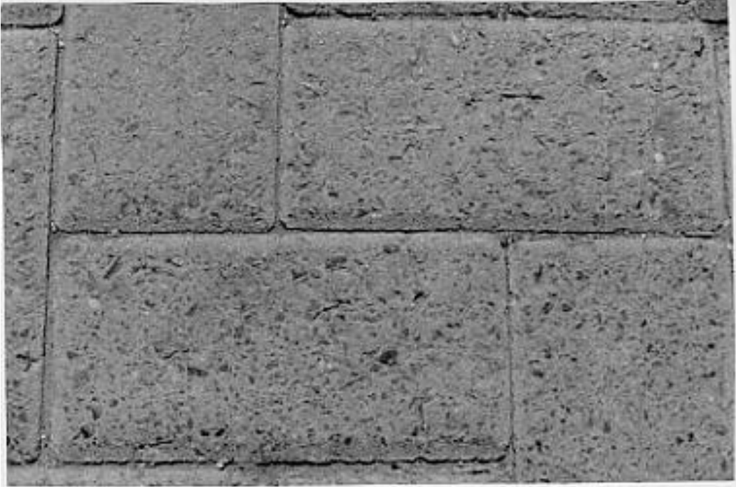
Figure 10.11 Example of aggregate protecting mortar component, Van Wyk Street, Roodepoort
