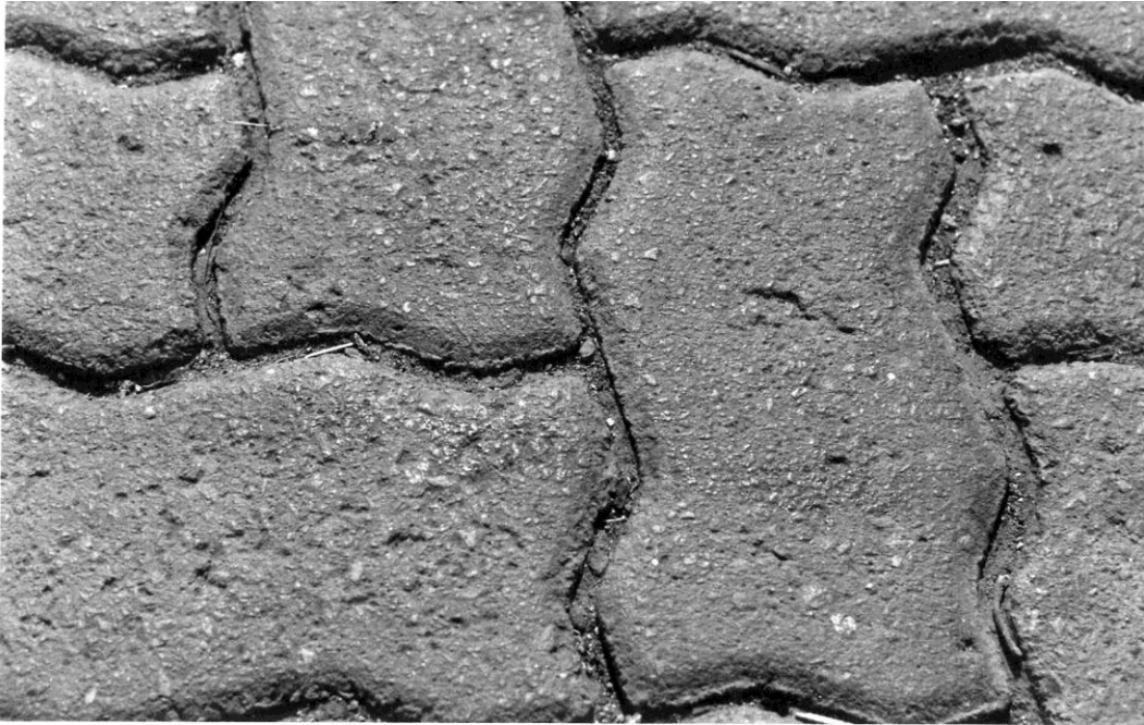
Figure 12.1 Polished appearance of high strength blocks after five years of traffic at Westgate. The blocks were made from high water and binder contents. The strong binder abrades only slightly faster than the aggregate, which takes the brunt of the attack.
