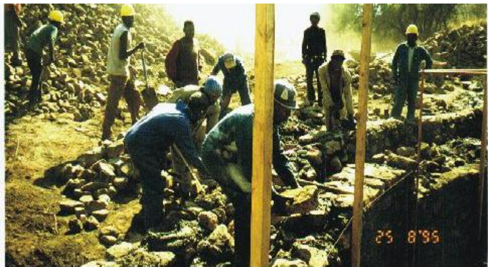
Figure 6 Example of a dam being constructed with RRC from rock that has been blasted. The tools are simple and the process is labour intensive.
