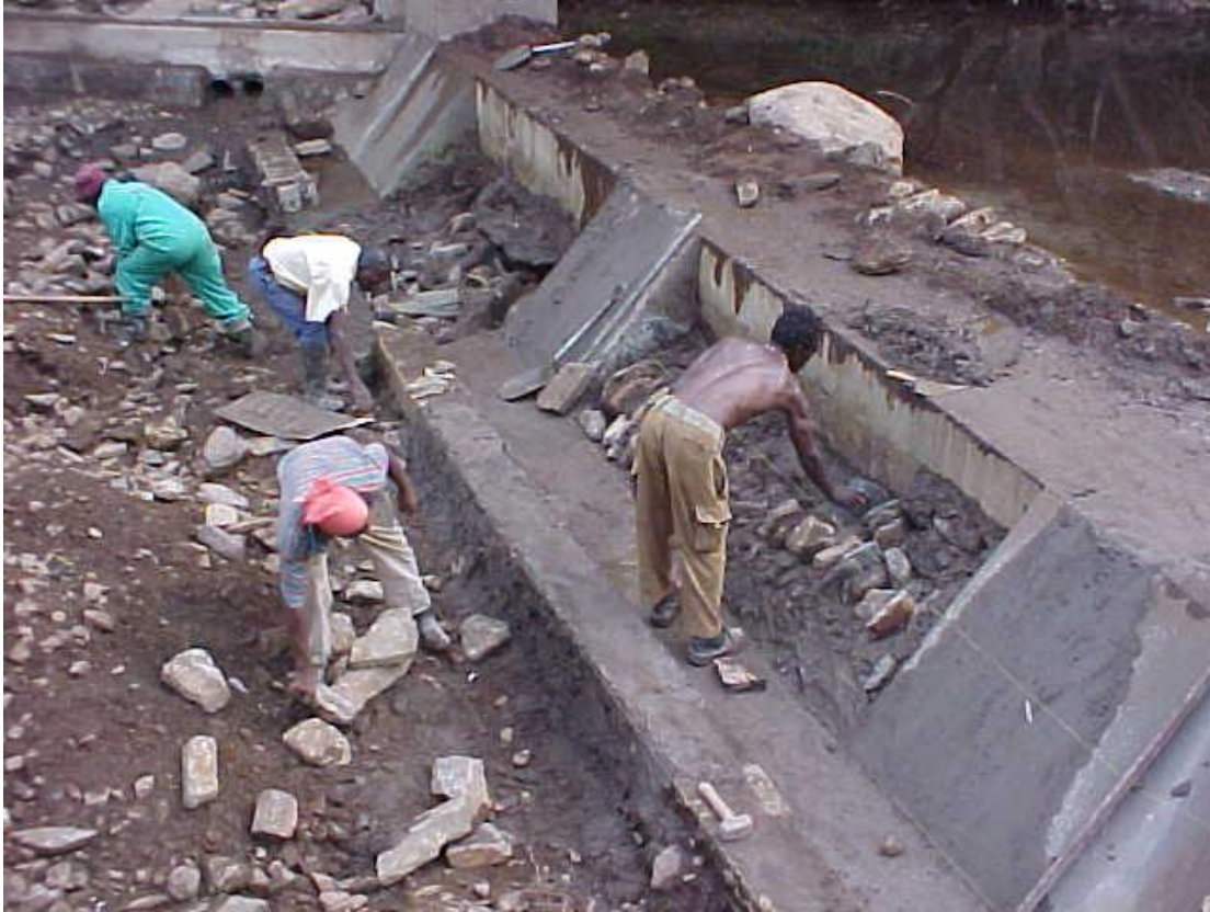
Figure 7 – Where ground is well consolidated it may be cost effective to construct the weir from a more rigid system such as random-rock-masonry as shown here. Much of the ground from which the re-engineered spillway is to be constructed is either undisturbed or well compacted, making this type of construction an option in the final design, if better suited than gabions. This diversion weir is situated in a gorge that has a 130km 2 catchment. (Designed and built – Dams for Africa 2003/4).
