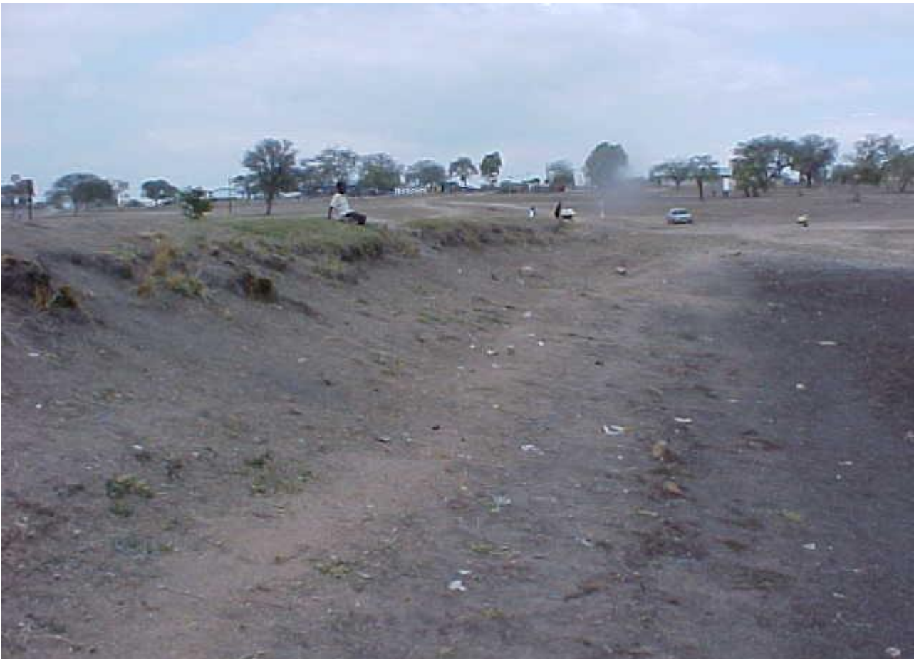
Figure 1 – A view of the Huntington community dam. The upstream embankment of this dam has noticeable erosion and there is evidence that it has been breached at one point, which implies an inadequate spillway. The reservoir is completely dry, which is not surprising given that it only has depth of 1.5m relative to the spillway.
