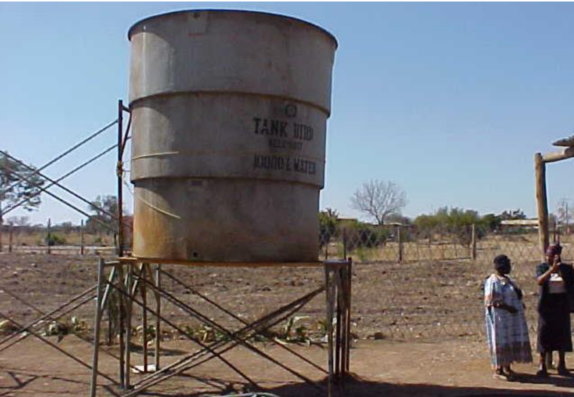
Figure 3 – View of existing 10000 litre tank
