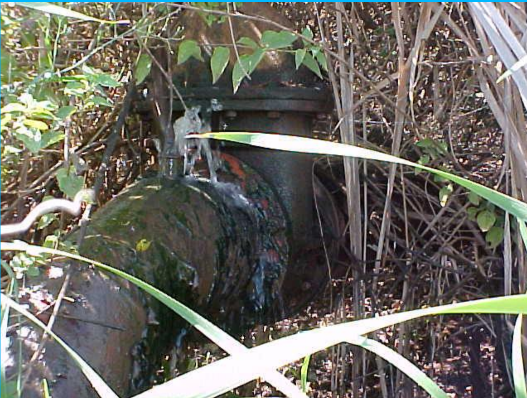
Figure 6 – View of 300mm outlet pipe as it exits in the embankment. By closing the main valve, it will be possible to cut a suitable hole in the pipe and weld on a 110mm coupling so that water may be piped to the fields as indicated in figure 7.
